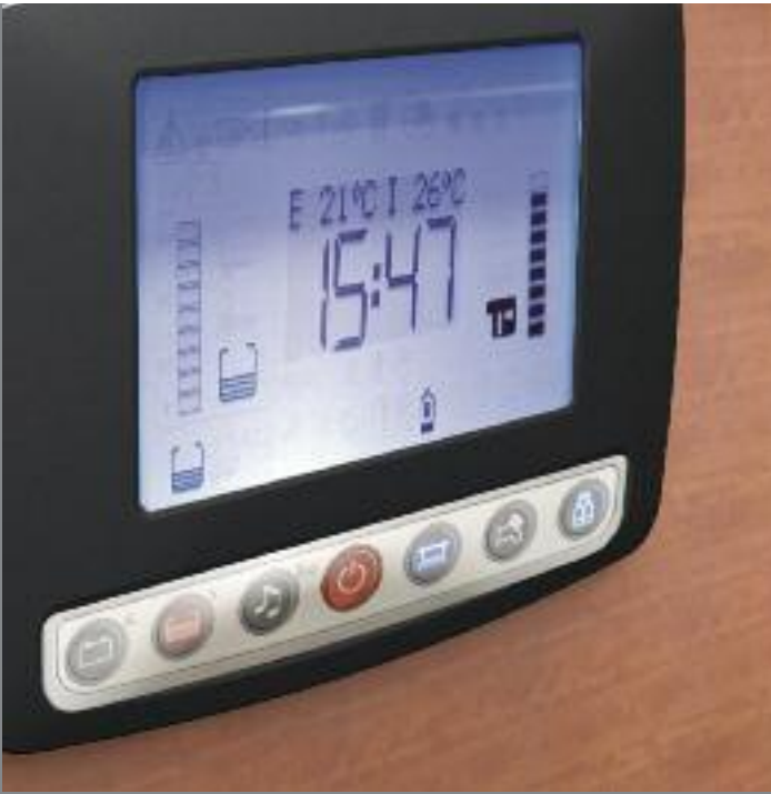
Technical control panel (not c-line)
